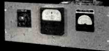
FREQUENCY MONITOR EXTENSION PANEL
